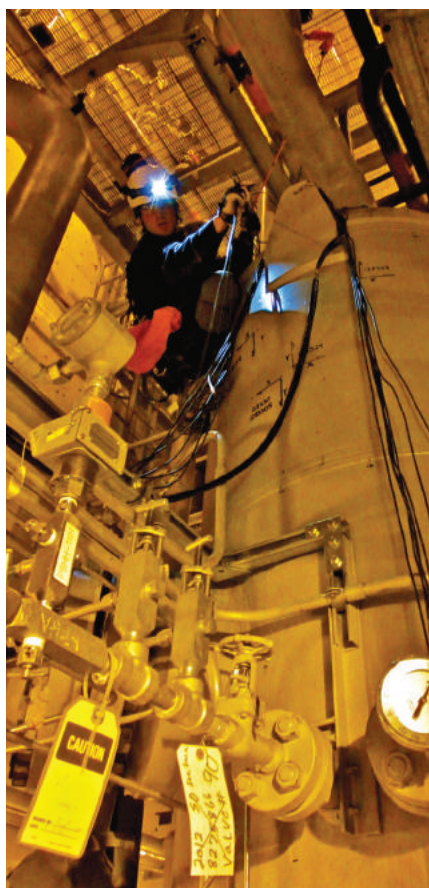
Tech11 in use in industrial rope access environment. Photo by Ben Erdman.
